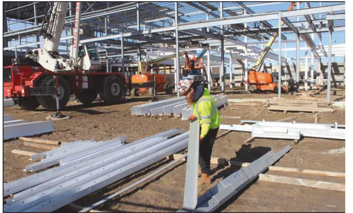
LIFTING A PIECE OF angle iron at the Harrison Street Commons project in Flint is Sean Dusek of Iron Workers Local 25. He’s employed by AMS Steel.
