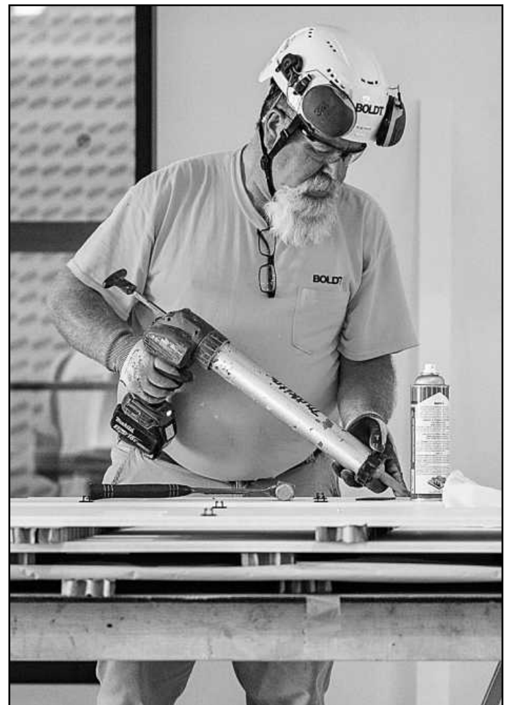
SAFETY HELMETS will be required of everyone on Boldt Co. jobsites by July 1. Hi-visibility clothing and safety glasses became mandated seemingly overnight about a decade ago on the nation's jobsites – time will tell if safety helmet requirements will become just as inevitable.
