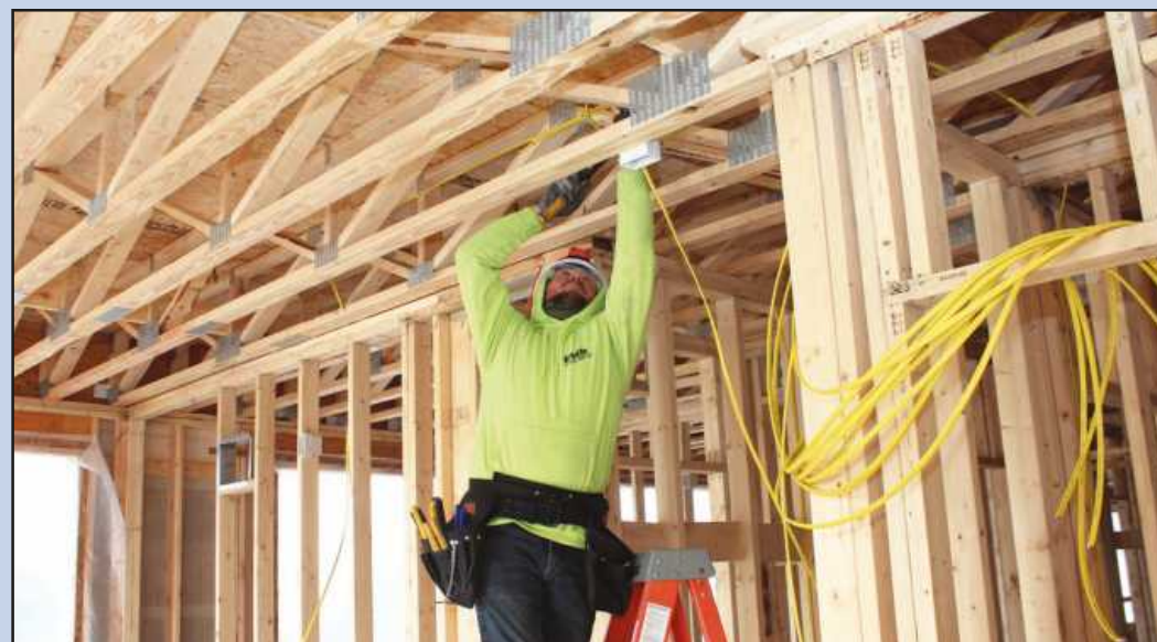
RUNNING NO. 12 WIRE in a fourth floor apartment at the Harrison Street Commons project in Flint is Marcos McDonald of IBEW Local 948. He's employed by Roth Electric.
