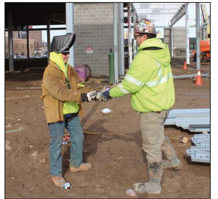
GETTING SOME CLIPS to be welded at the Harrison Street Commons project in Flint are iron worker journeyman Tanya Curtis. Handing them to her are foreman Troy Breasbois. The Local 25 members are working for AMS Steel.
