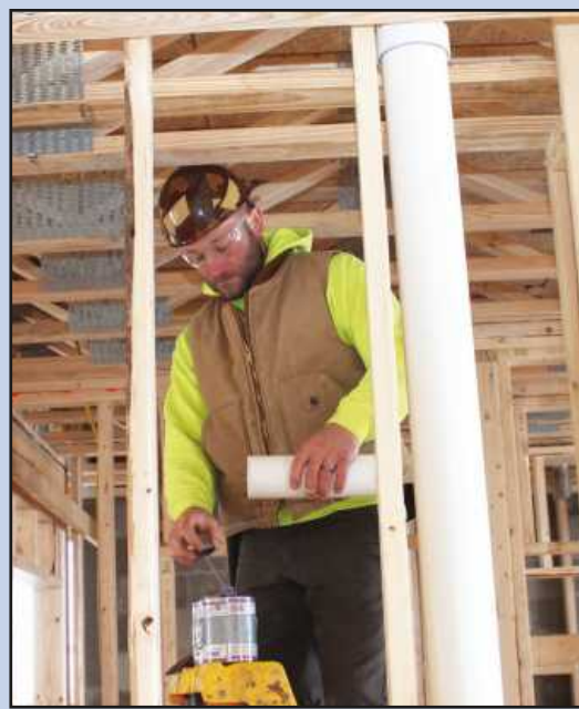
APPLYING PVC CEMENT to a three-inch drain pipe in a third floor apartment at the Harrison Street Commons project in Flint is Jesse Nickels. The Plumbers and Pipe Fitters Local 370 member is employed by Goyette.
