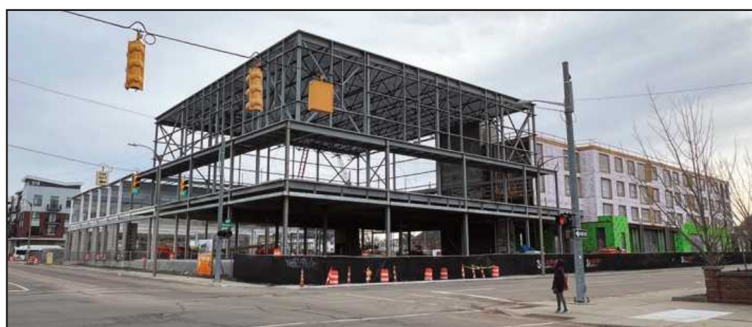
GOING UP at Harrison and Third Streets in Flint: the Harrison Street Commons project, which combines a YMCA with 50 apartments.
