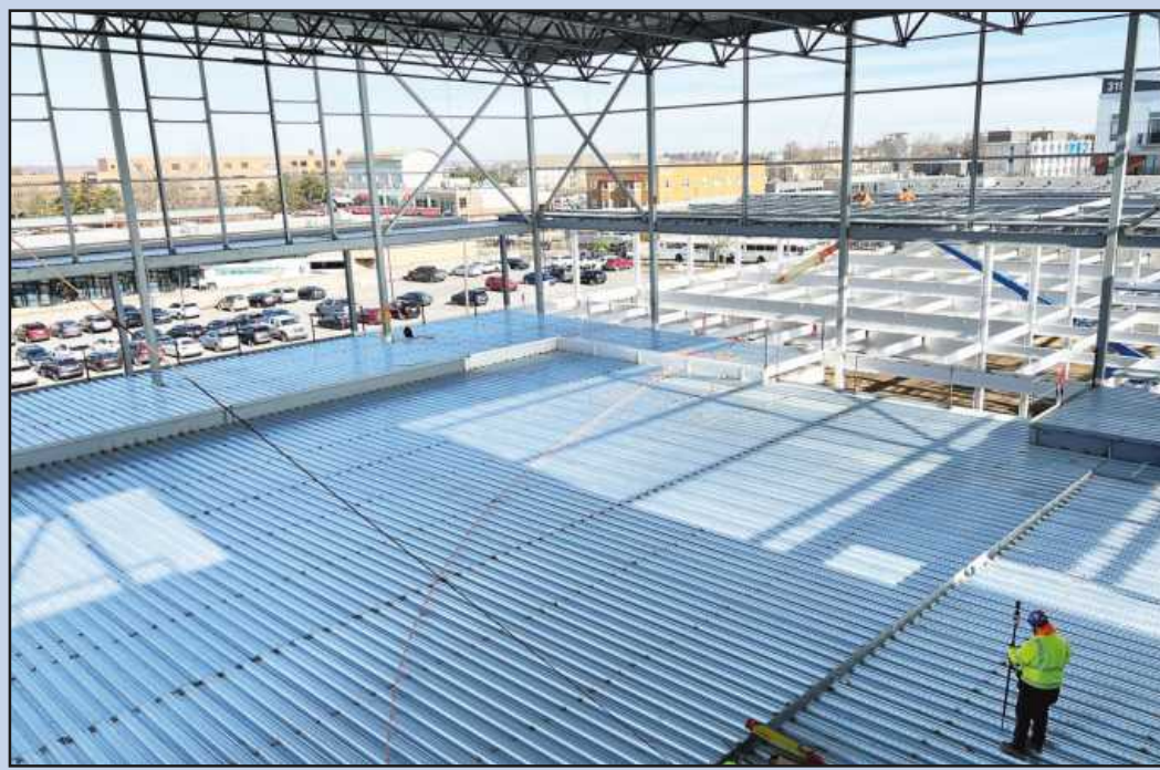
USING A "Total Station" precision scanner to set the locations for duct hangers on the floor below is Colby Hengesberg of Sheet Metal Workers Local 7. Employed by Dee Cramer, he's working on the YMCA portion of the Harrison Street Commons project in an area that will have a basketball court and running track.
